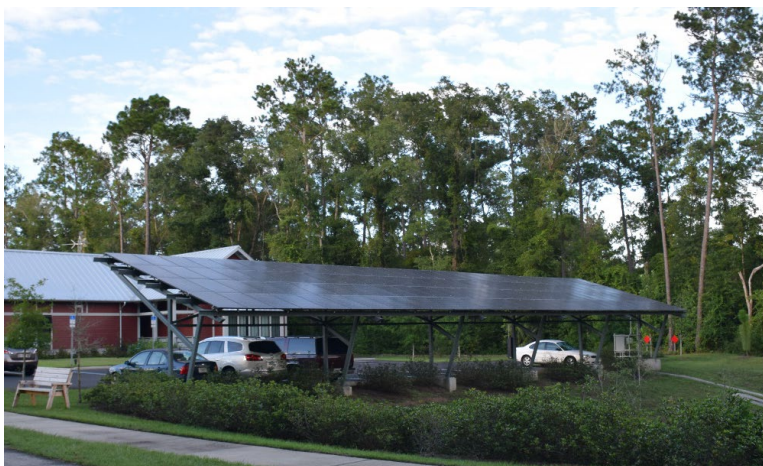
Figure 49. Solar EV charging canopy at the Dwellings sustainable housing development in Tallahassee, Florida (photo: R. Meeker, Nhu Energy).
