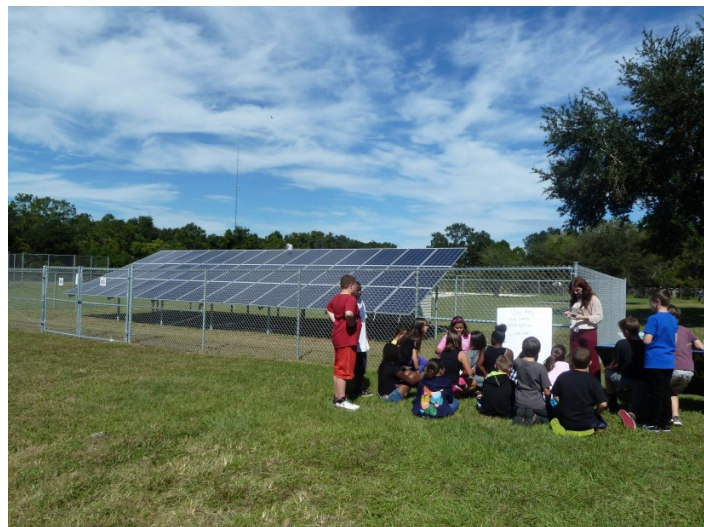
Figure 90. Through the SunSmart Schools and Emergency Shelters Program, over 106 schools in Florida have solar PV + battery energy storage systems (photo by Amy Kidd) [185].
