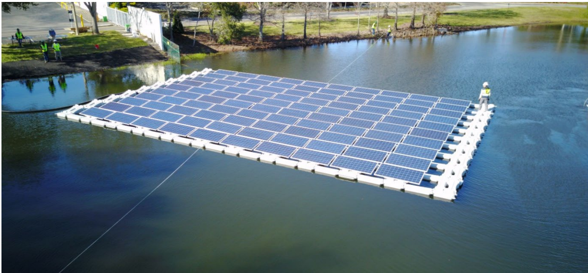
Figure 46. A 31.5 kW AC floating solar array installed in 2017 at Orlando Utility Commission's (OUC's) Gardenia Operations Center in Orlando, FL. In 2020, the system was expanded to 59.2 kW AC . (photo courtesy J. Kramer, OUC)
